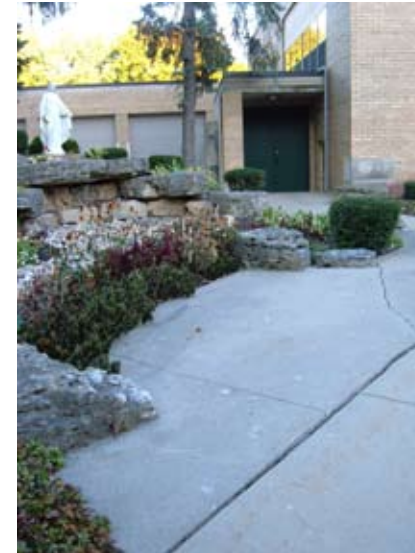
A dedication/memorial walk will replace cracked and heaved concrete in front of the Blessed Virgin Mary garden.
