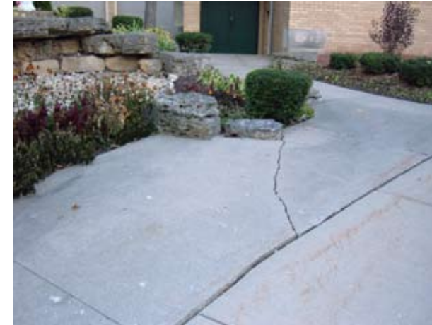
Before Project - cracked & raised concrete
